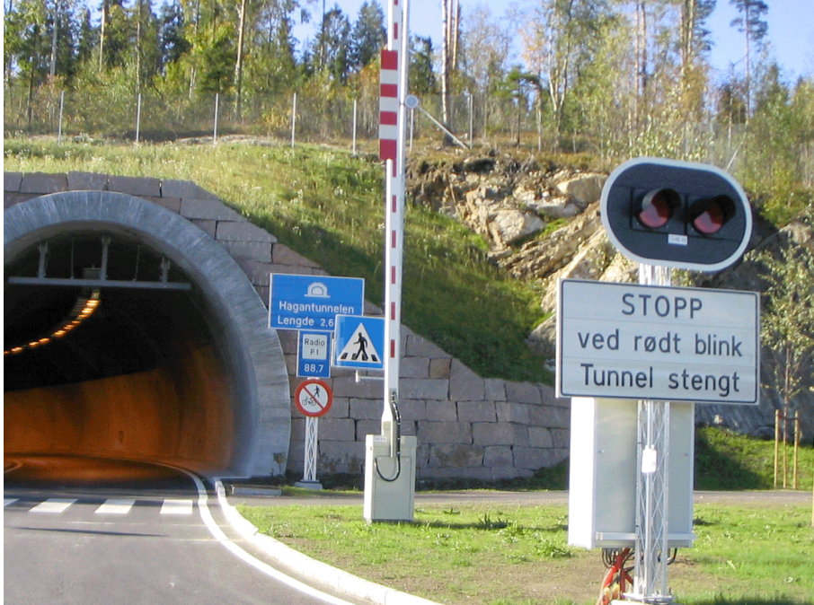
The I/O cabinet also includes an Ethernet Switch. This is located in the cabinet below the red signal light
